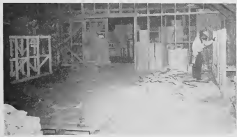
The building which will hold the pickup and delivery section of the commissary is rapidly reconditioned. Here a workman tears out old storage racks. The windows will be used for pickup windows; shelving and wiring are also being installed.
